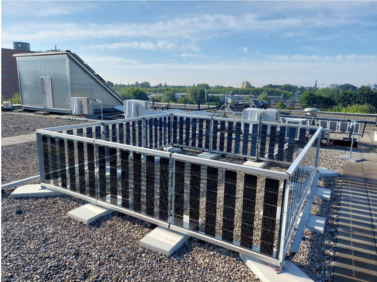
Figure 4: Bifacial PV Terrace Fence in 4 different orientations (3 prototypes per orientation). Can also be implemented as a balcony.
